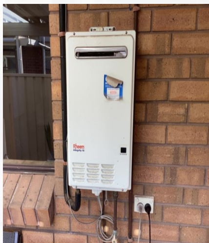
Old Rheem instantaneous gas hot water unit
